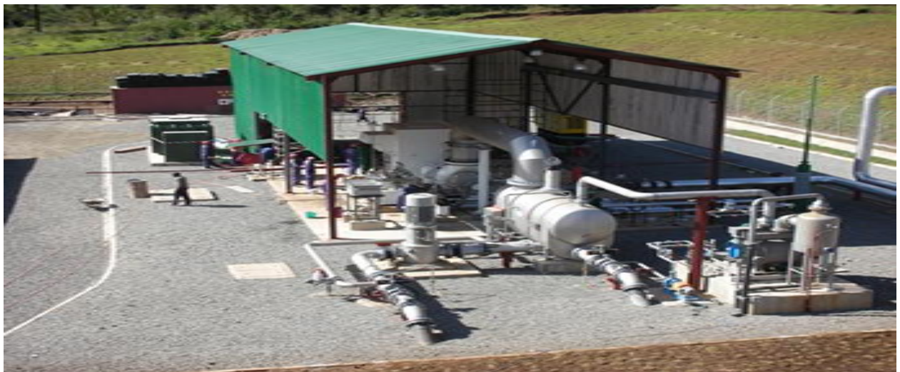
Figure 1: Eburru 2.4 MW wellhead power plant [38]
